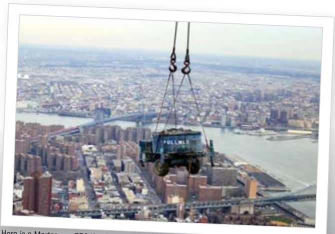
Here is a Mortarman 750 that is being lifted by helicopter to the top of the Freedom Tower in NYC. From the roof of the Tower a beautiful spire goes up and up, the Mortarman 750 mixed the specialty grout that holds the spire in place. - Thanks to Bill Drudy, RFI Construction Products, Farmingdale, NY.
